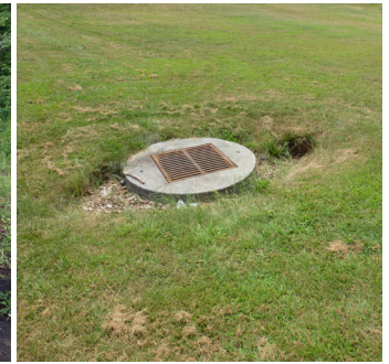
Series of drop inlets through park with evidence of some settling.
